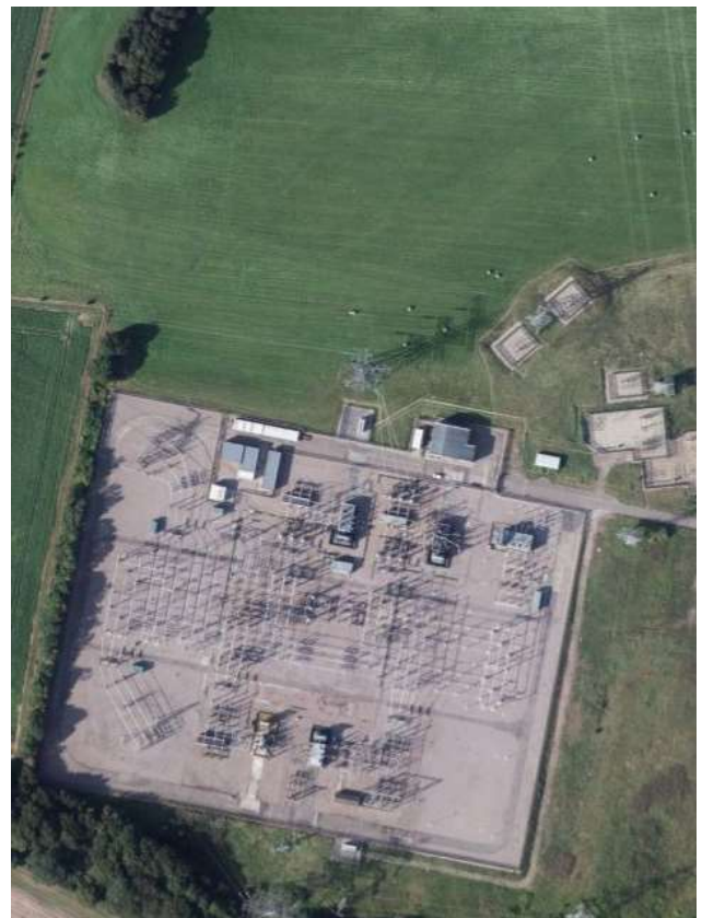
Dunston Woods substation
